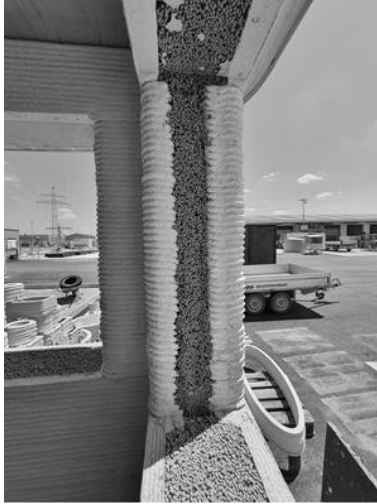
Fig. 1 insulation in the wall cavity (source: Andrea Palazzo 3D wall by Rupp Gebäudedruck)
